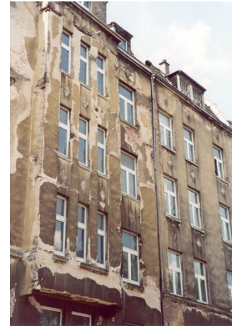
War damages on houses still in 2004
